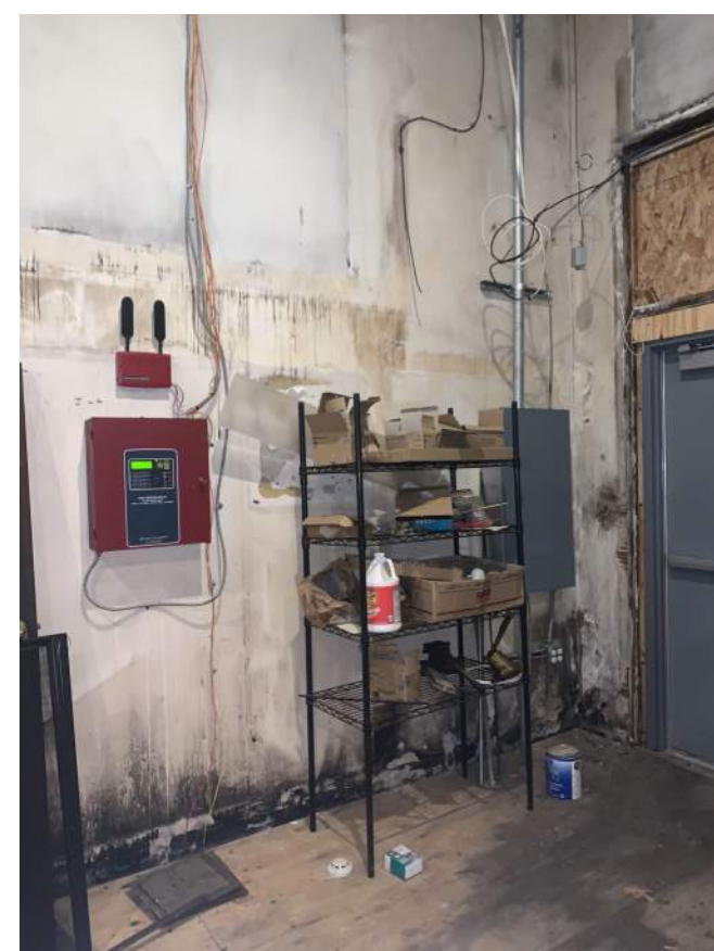
5 FIRE & ELECTRICAL PANELS Future Barber Shop
