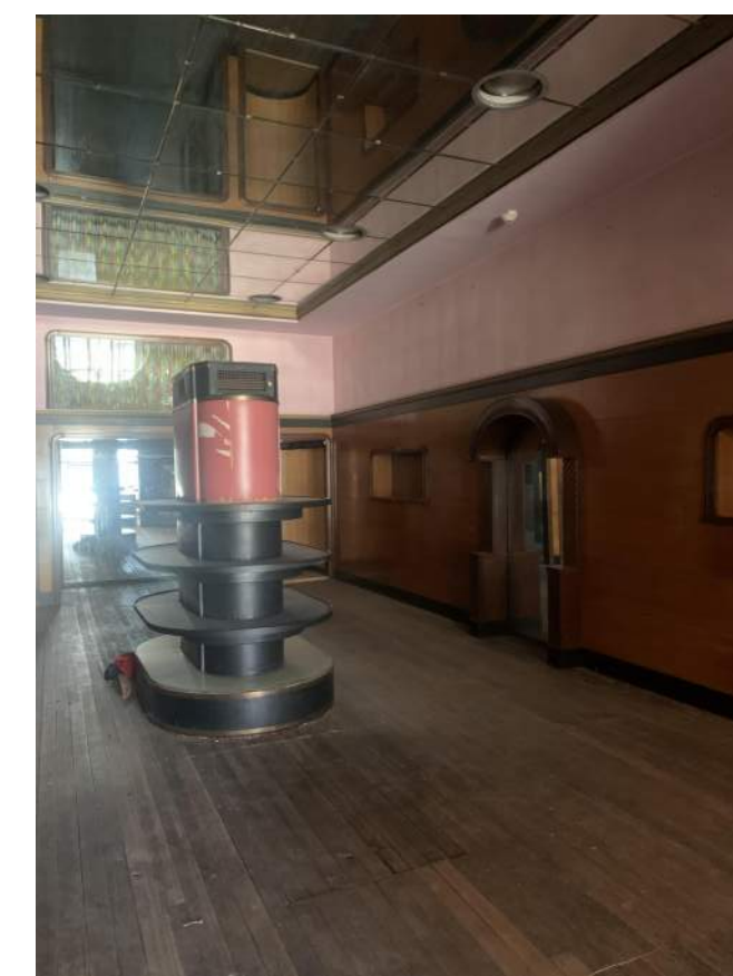
7 EXISTING AIR EQUIP./ NORTH WALL Future Men's Store
